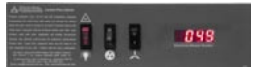
Control Panel with a 3-way switch for UV and fluorescent light
